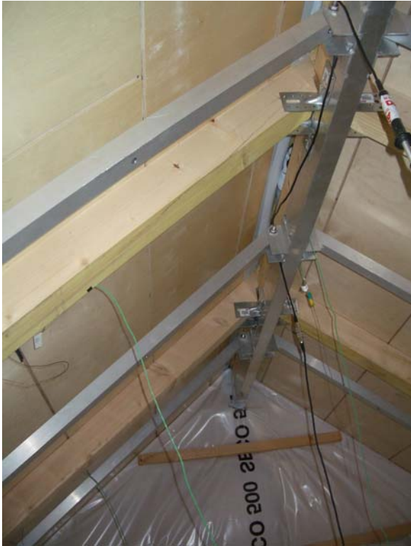
Picture 5: Interior view of the roof according to the thermography picture
